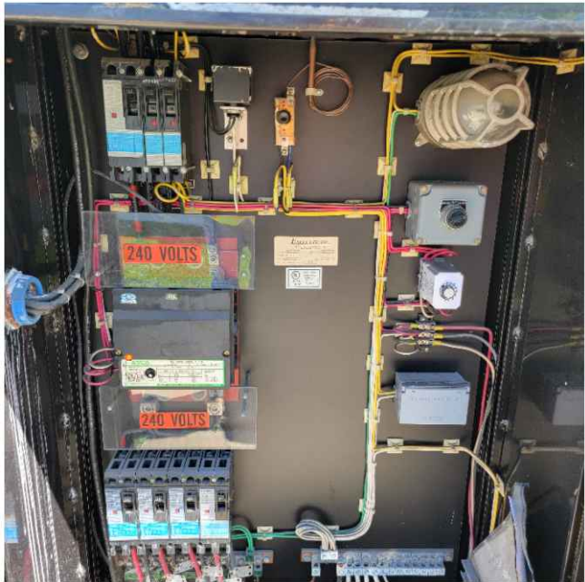
EXISTING LIGHTING CONTROLLER
