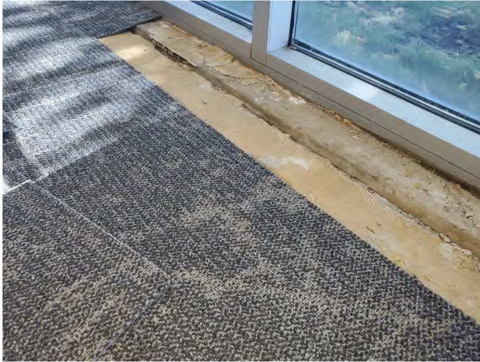
Photograph 1. Vertical displacement of the floor slab with respect to the concrete foundation wall along the southern exterior wall of the structure.
