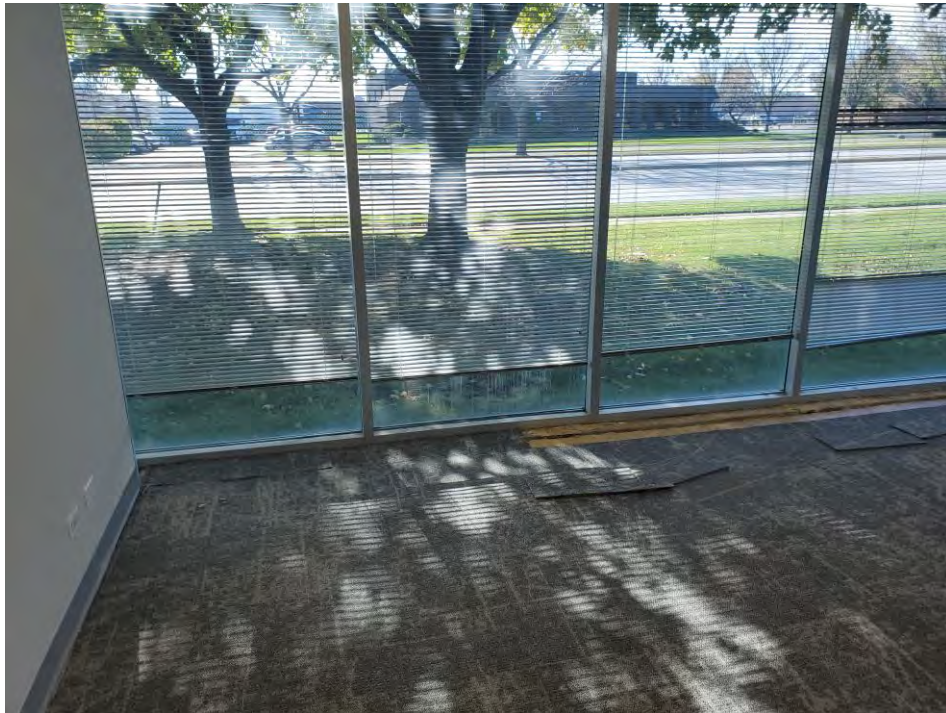
Photograph 3. A tree was present at the exterior coincident with the slab displacement.
