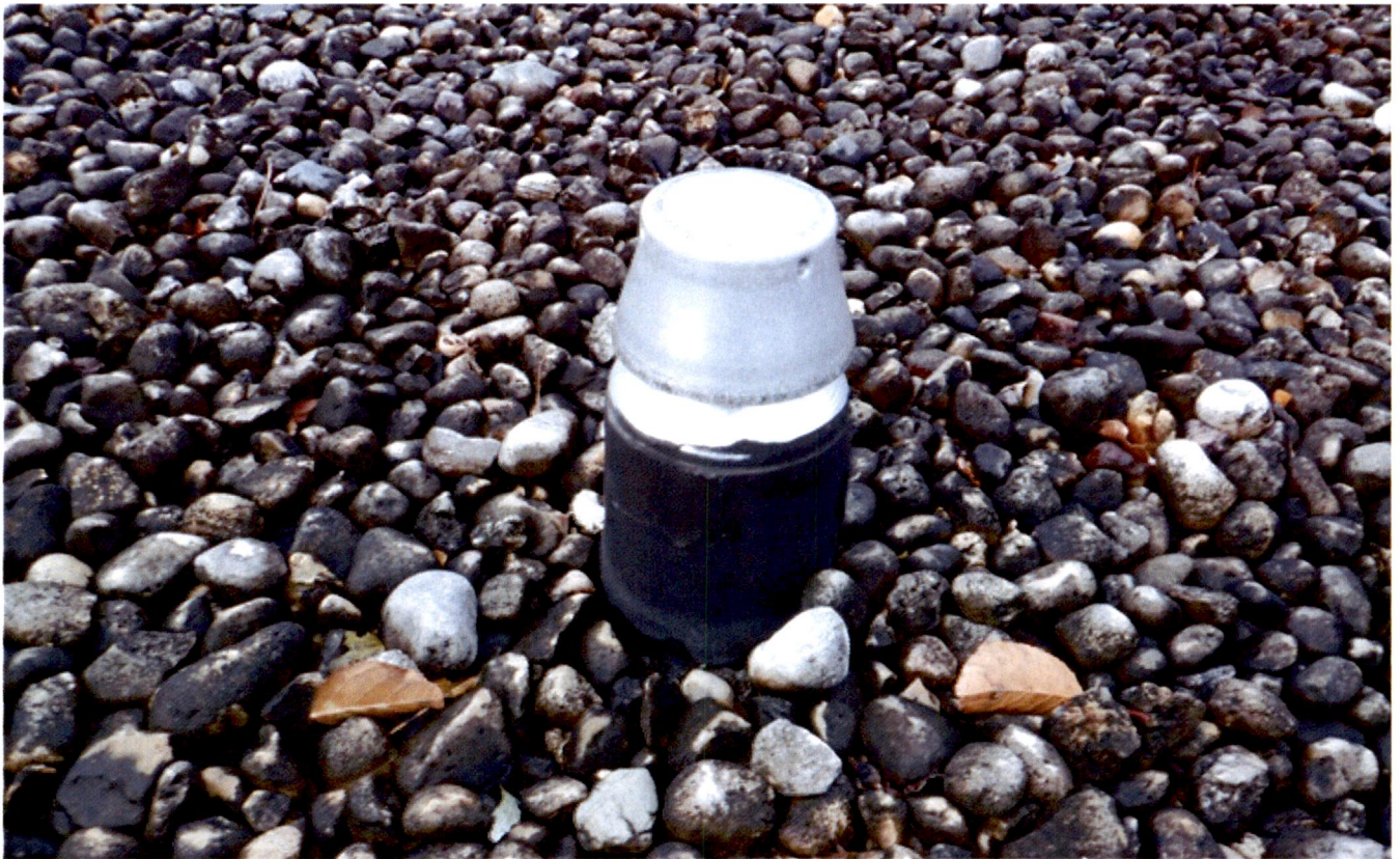
9. Vent for rubber roof membrane.
