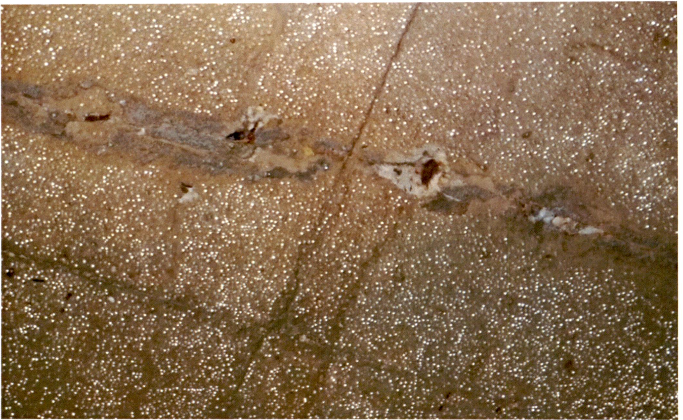
29. Cracks in roof and exposed rebar.
