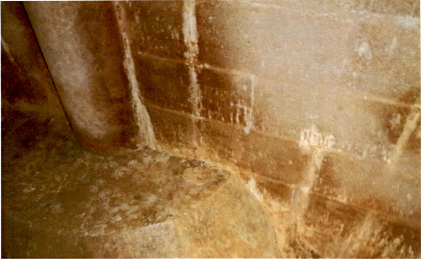
53. Efflorescence at cracks in baffle wall.
