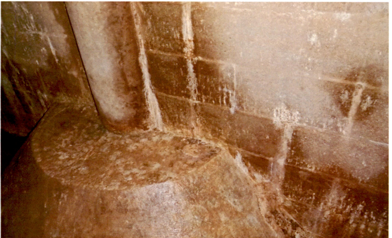
52. Efflorescence at cracks in baffle wall.
