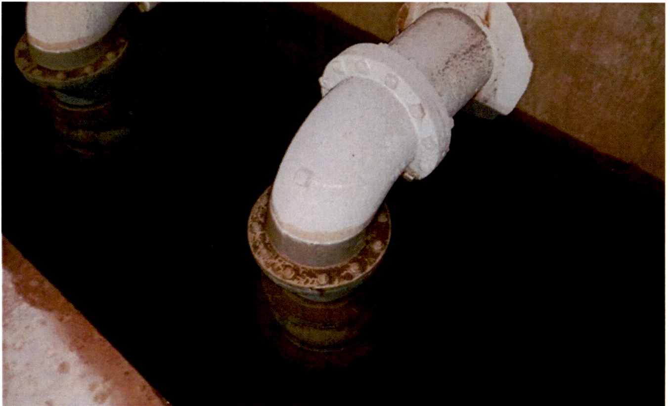
64. Piping in sump.
