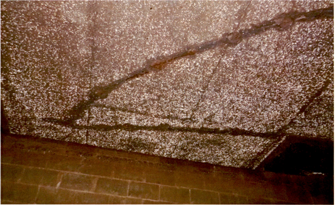
31. Cracks in roof at baffle wall.
