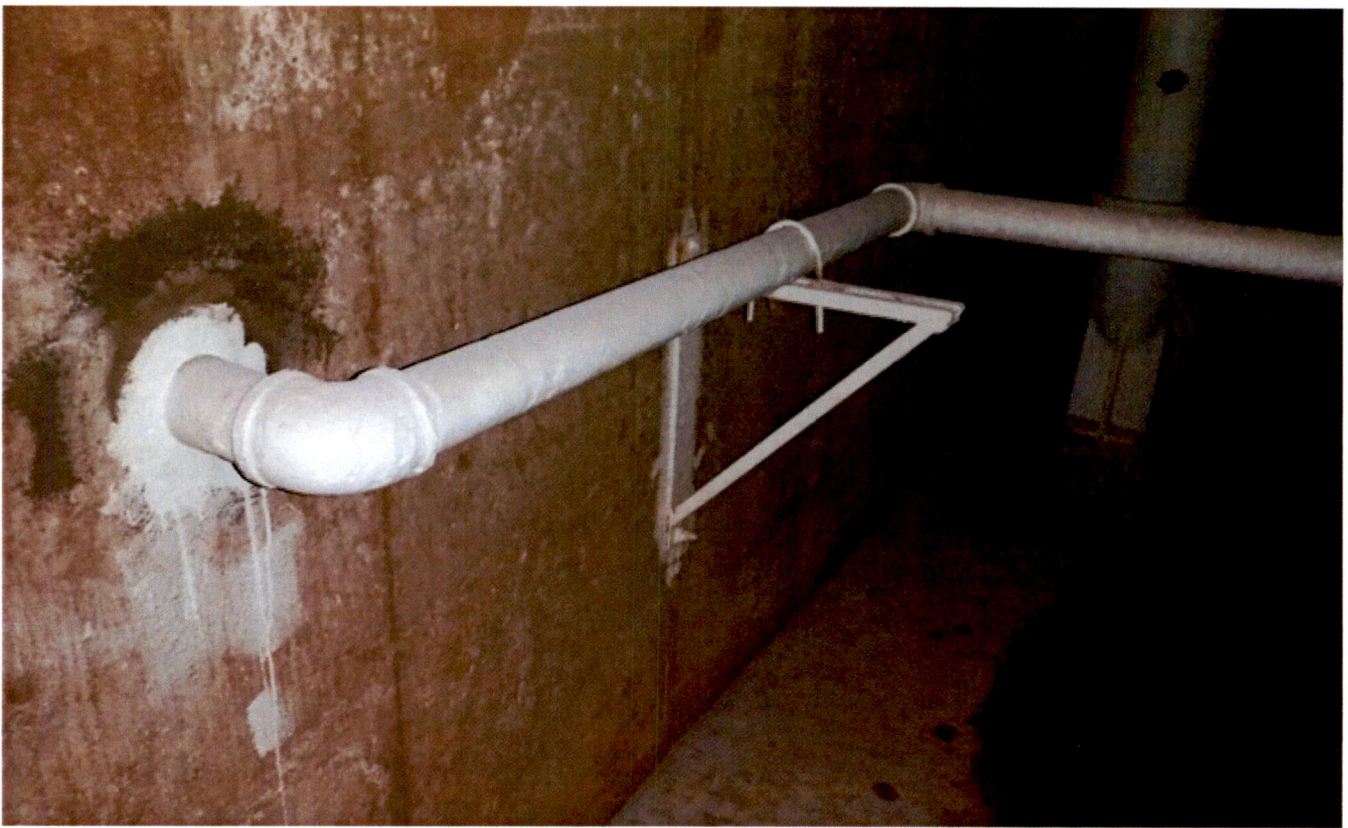
60. Interior piping and pipe bracket.
