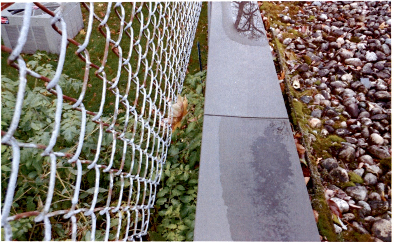
19. Water ponded adjacent to roof manhole.
