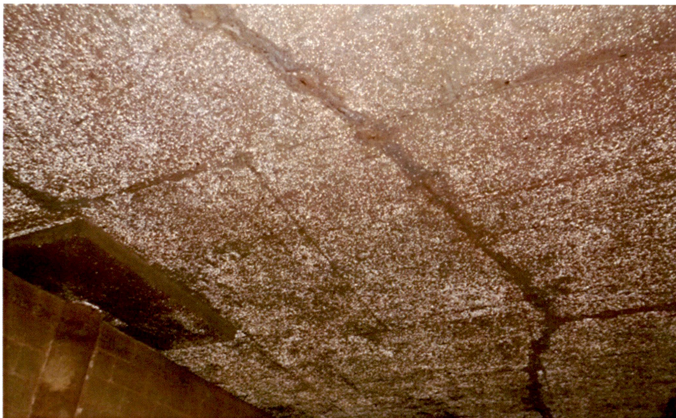
35. Cracks and exposed rebar in roof adjacent to baffle wall.
