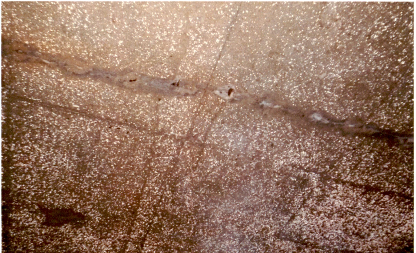
28. Cracks in roof and exposed rebar.
