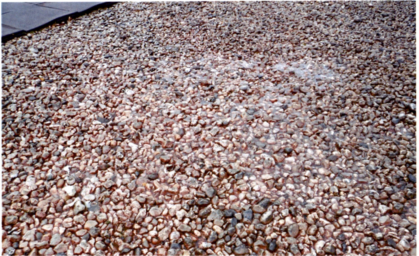
15. Ponded water on roof.
