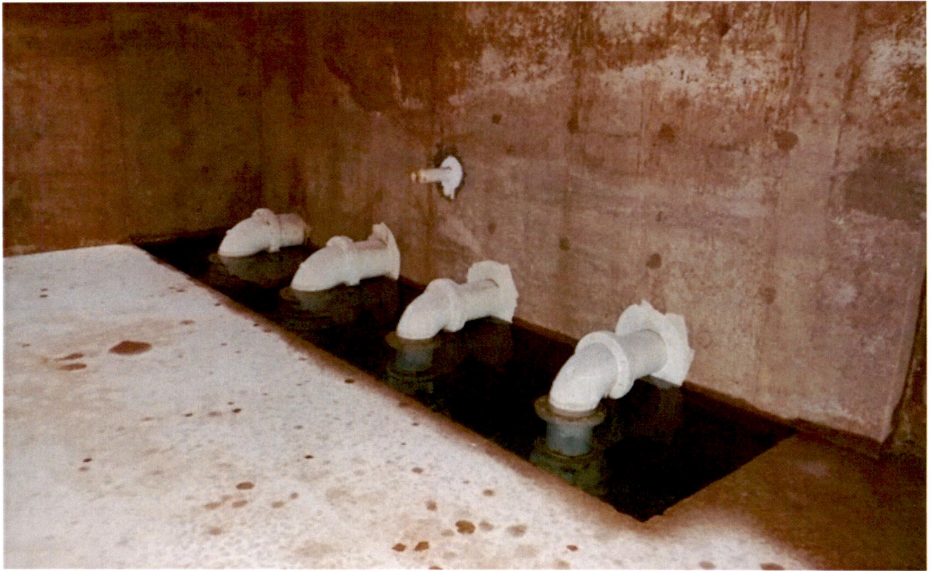
63. Sump in floor and interior piping.
