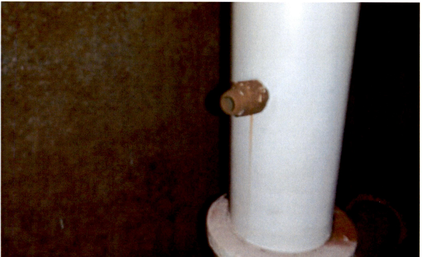
62. Coupling penetration in interior pipe.
