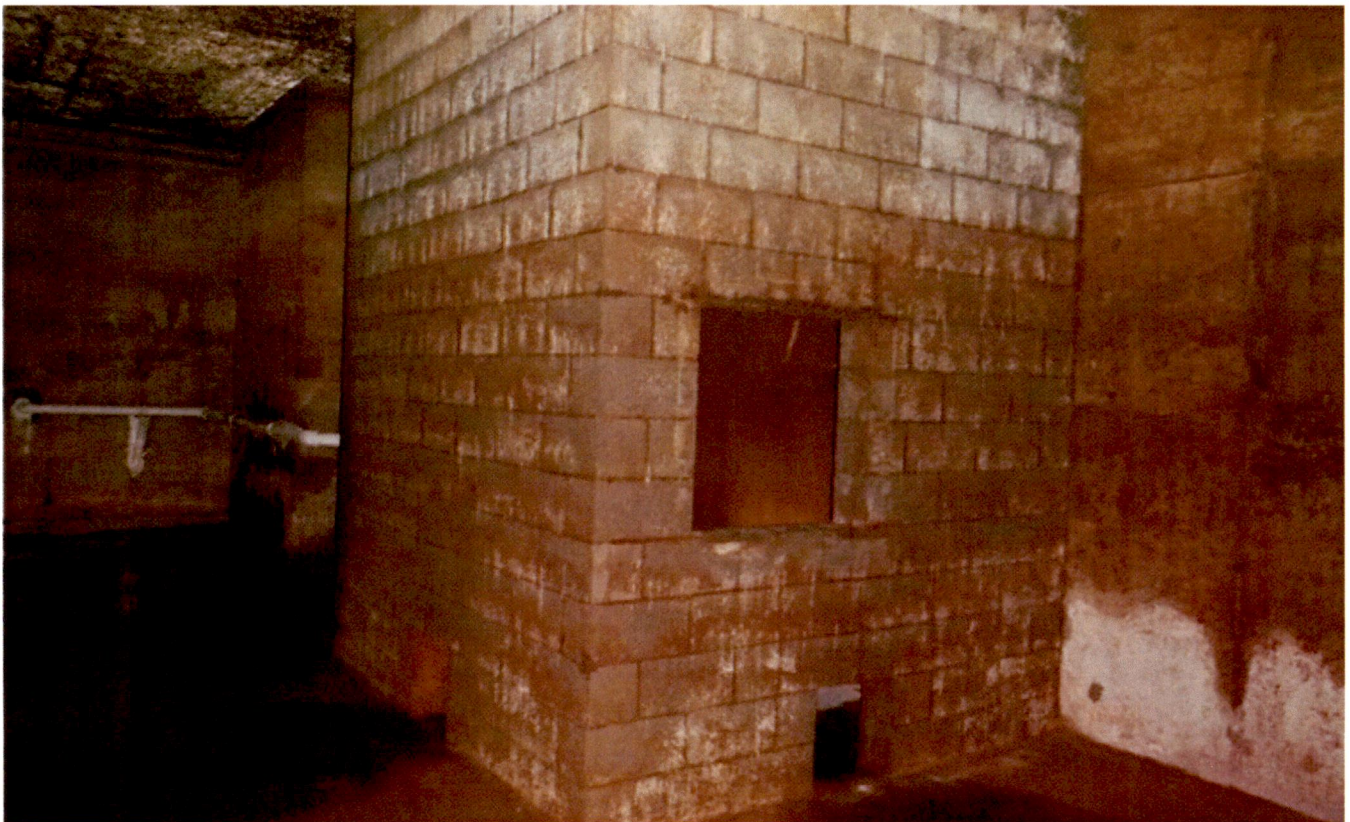
42. Openings in baffle wall.
