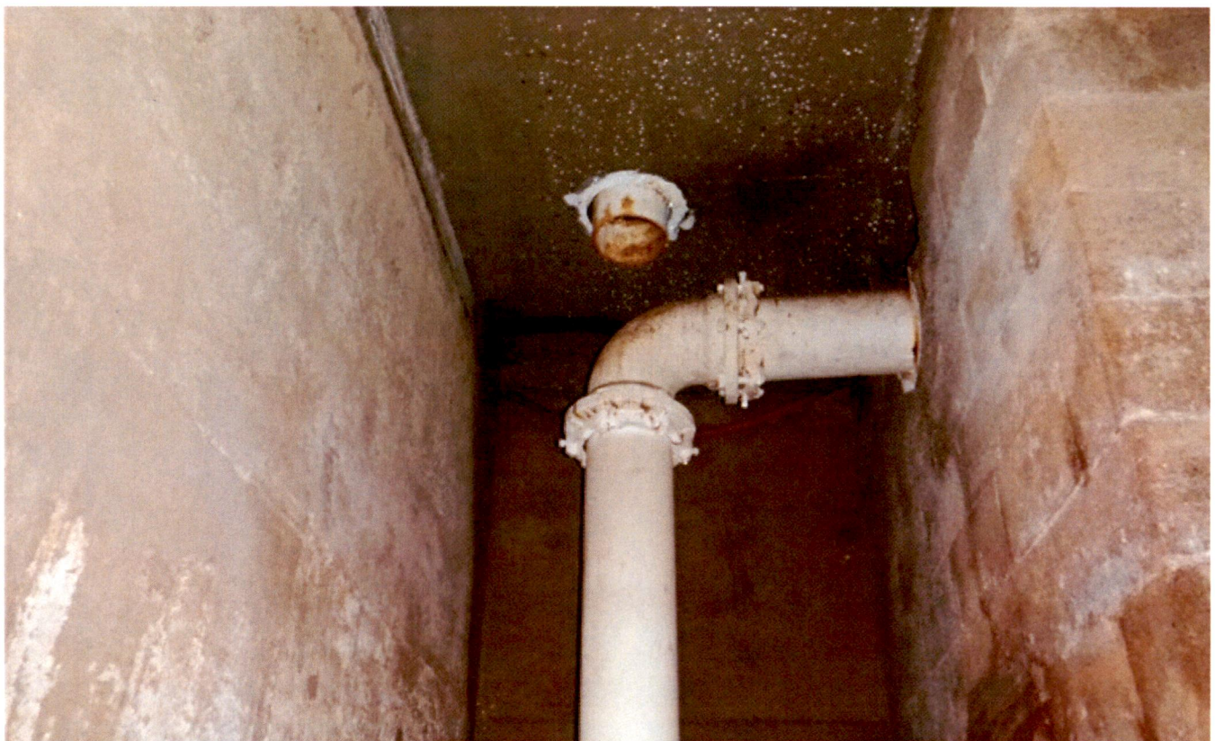
58. Pipe penetration in roof and interior piping.
