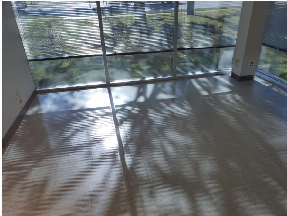
Photograph 4. Vertical slab displacement was also apparent at the southwest corner of the structure. Note the large tree at the exterior.
