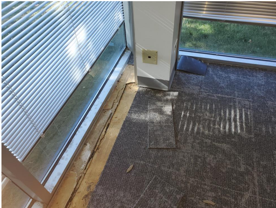
Photograph 2. The vertical displacement was apparent between the base trim around the column and the carpet.
