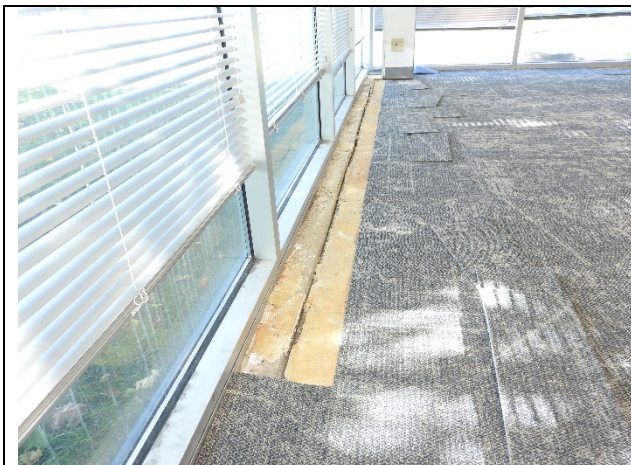
Photo 1: Depicts slab displacement along the east office wall looking south.
