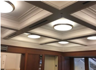
VH interior lighting retrofit
