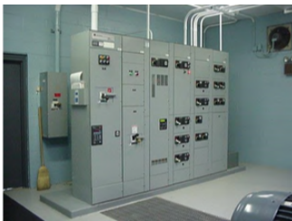
Motor Control Center that houses VFD's
