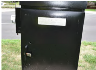
Street Light Control Cabinet
