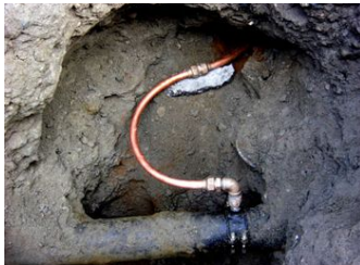
Copper Service Line Connection
