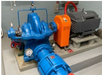
High Service Booster Pump
