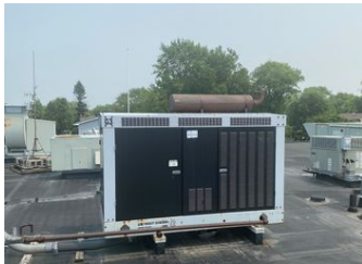
Fire Station 12 Generator
